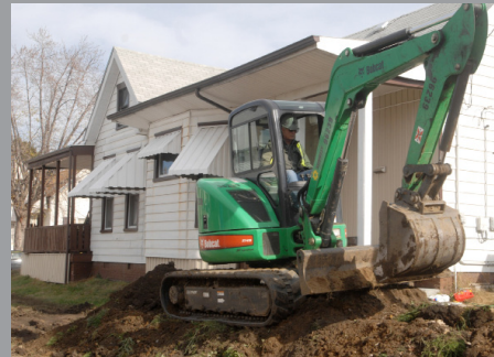
The EPA cleanup consisted of contractors coming into contaminated yards and replacing the soil using heavy machinery.
