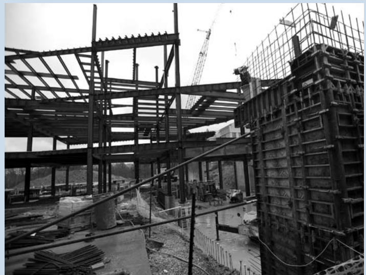
Steel framework of the new Business and Engineering Center is rising. The building is due for completion in fall 2010.
