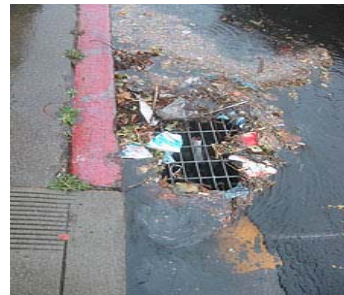
Trash at drain
